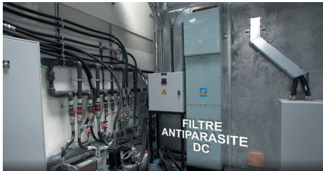
The MPE TEMPEST power line filter in situ
